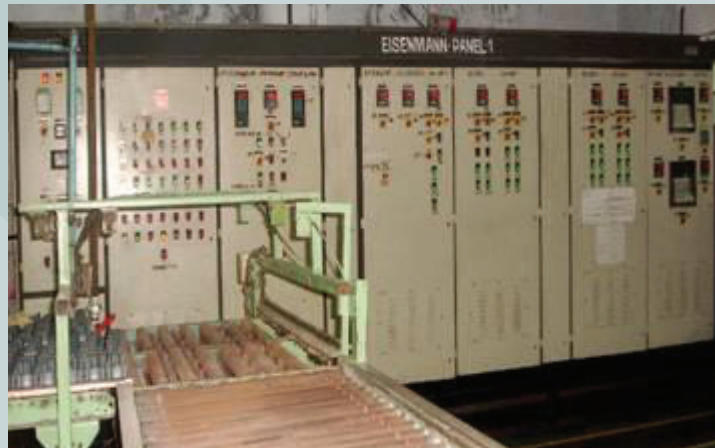
Logic controllers for total control of Sintering cycle
